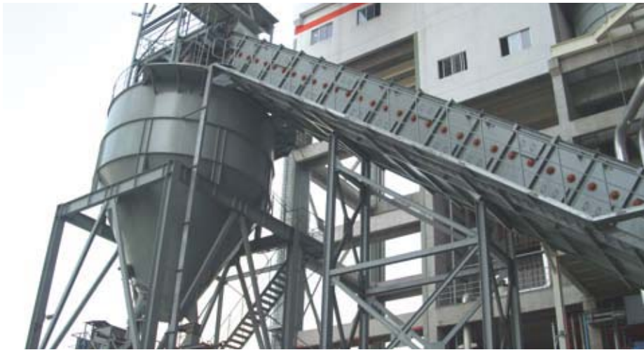
Typical Clyde Bergemann DRYCON system conveying to a silo
