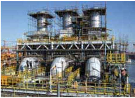
Three WHRU installed on Modec's Guara FPSO
