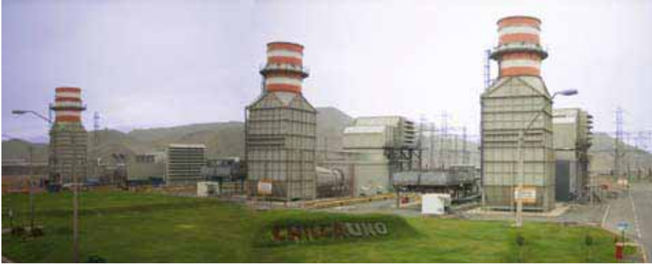
Existing gas turbine exhaust stacks at the Chilca Uno power plant, Peru
