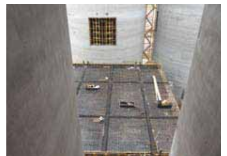
Conditioner building within the fly ash silos
