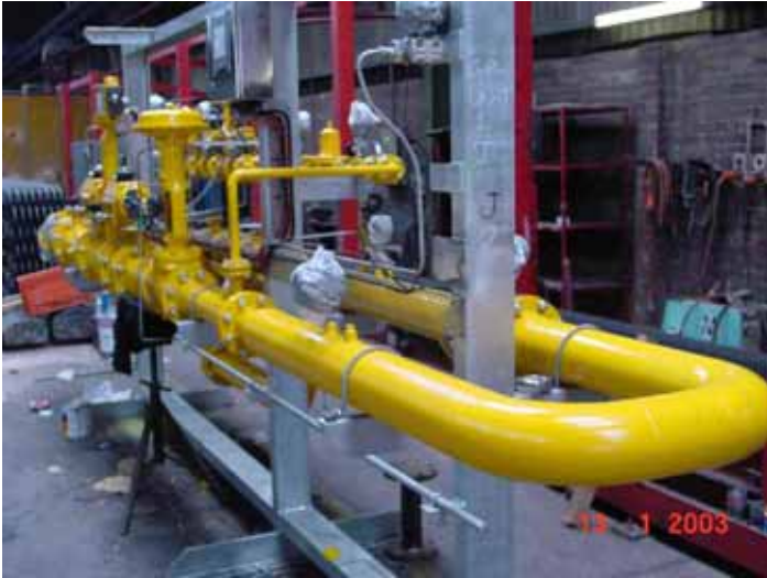
Gas Skid Assembly
