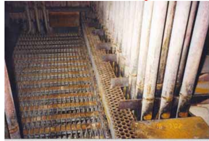
Installed On Site – By Others
